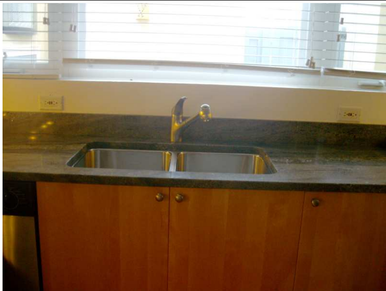
KOHLER Stainless steel double sink with an American Standard faucet
